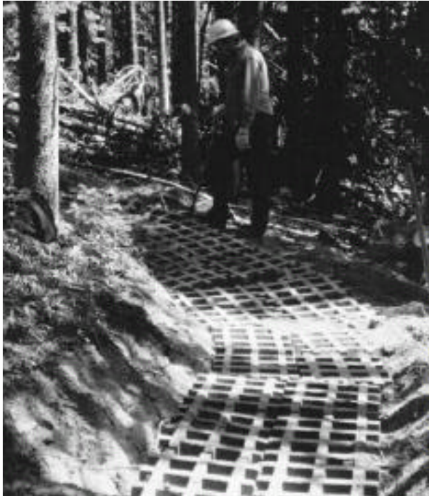
Figure 5. Concrete blocks, installed in a trail to reduce erosion from dirtbikes, make for awkward footing for pedestrians. This installation on public land was funded out of Washington State gasoline taxes. Photo: Washington Interagency Committee for Outdoor Recreation.
